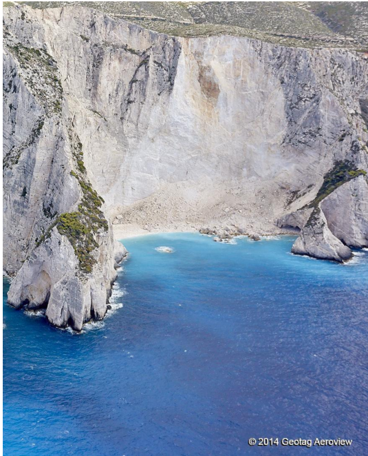
(a) Zakyntos cliffs erosion (Shipwreck beach, Greece)
