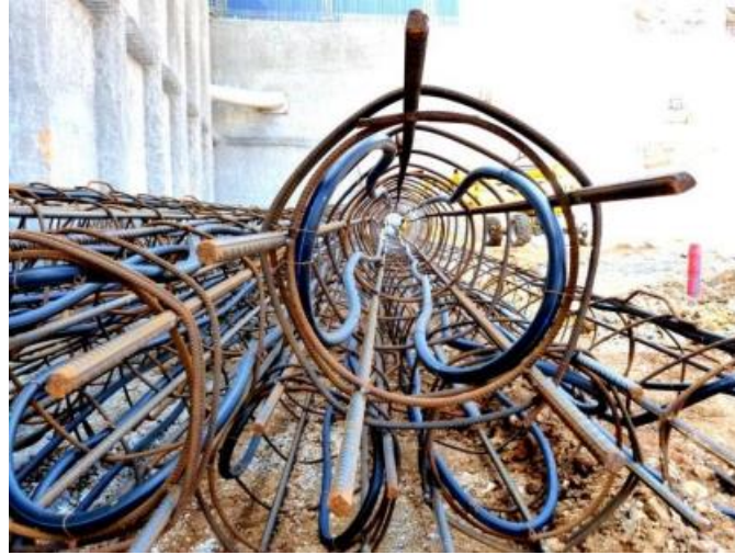
Figure I. 12 - Illustration of the fixing of HDPE pipes on energy pile reinforcement (geothermie-professionnelle)
