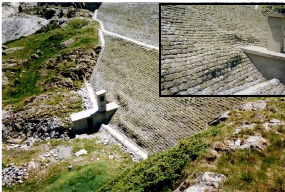
Fig. I.10. Bulges observed on the downstream pitching of Escoubous dam (©EDF)
