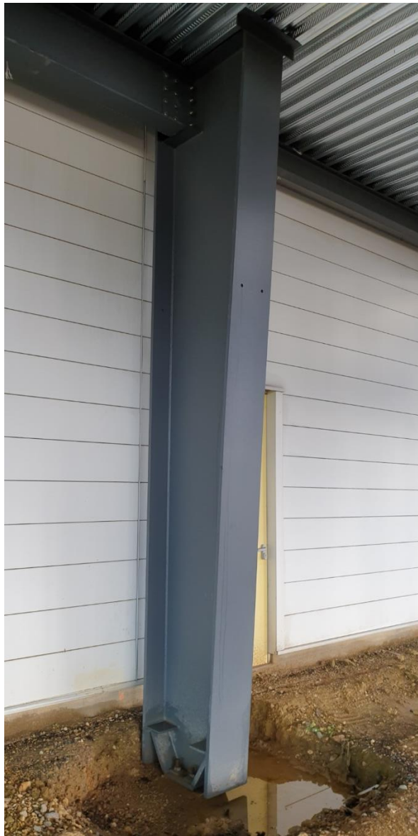
Figure I-1: Tapered column in a steel building (Lisses (91), France)
