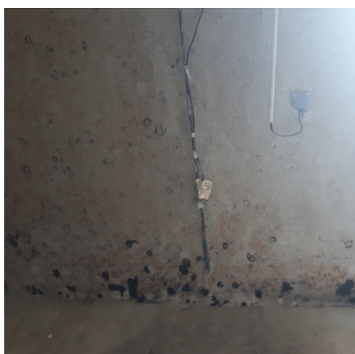
Figure 106. In situ mold proliferation on inside insulation hemp mortar
