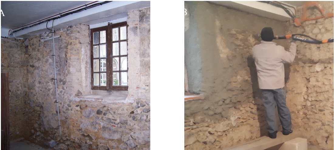
Figure 104. Image of the wall before the hemp mortar insulation (a) and the application process (b)
