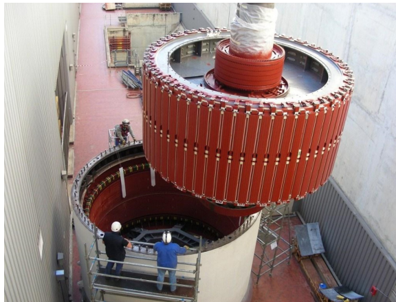
Figure 7.1 – Photo of a turbine undergoing maintenance. The rotor is extracted from the stator in this operation. Source: CNR.
