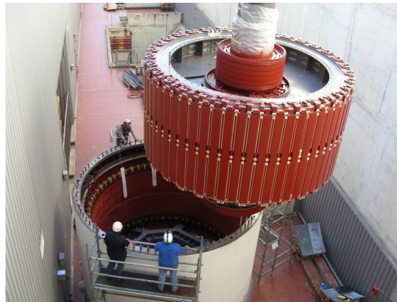
Figure 7.1 – Photo of a turbine undergoing maintenance. The rotor is extracted from the stator in this operation. Source: CNR.
