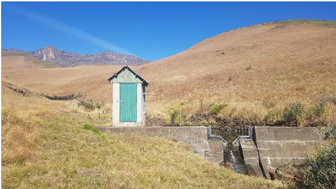
Figure 3.2: Concrete weir and stilling hut, with 90-degree V Notch installed at CP-VI
