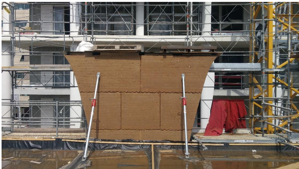
Figure 4.59: Pictures showing the assembled prefabricated blocks of an element of wall (source: author)
