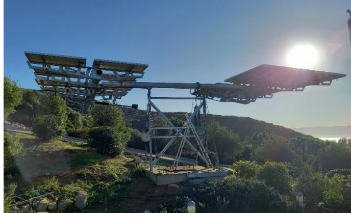
Figure 3-7: The PV tracker in its “rest” position
