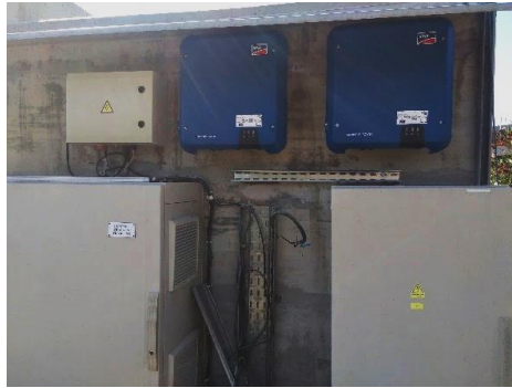
Figure 3-12: Inverters and instrumentation panels
