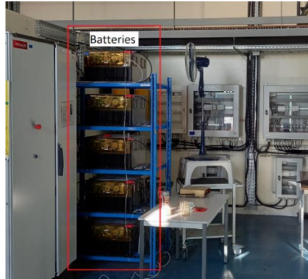
Figure 3-2: View of one of the battery banks (Zebra batteries) inside the powerhouse
