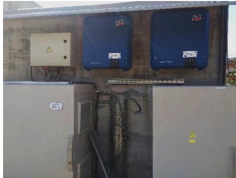
Figure 3-12: Inverters and instrumentation panels
