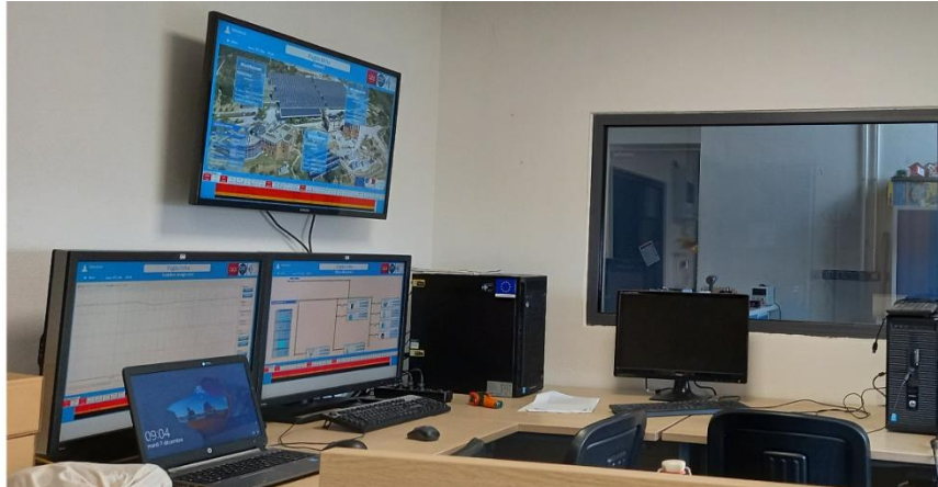
Figure 3-5: The control room inside the powerhouse
