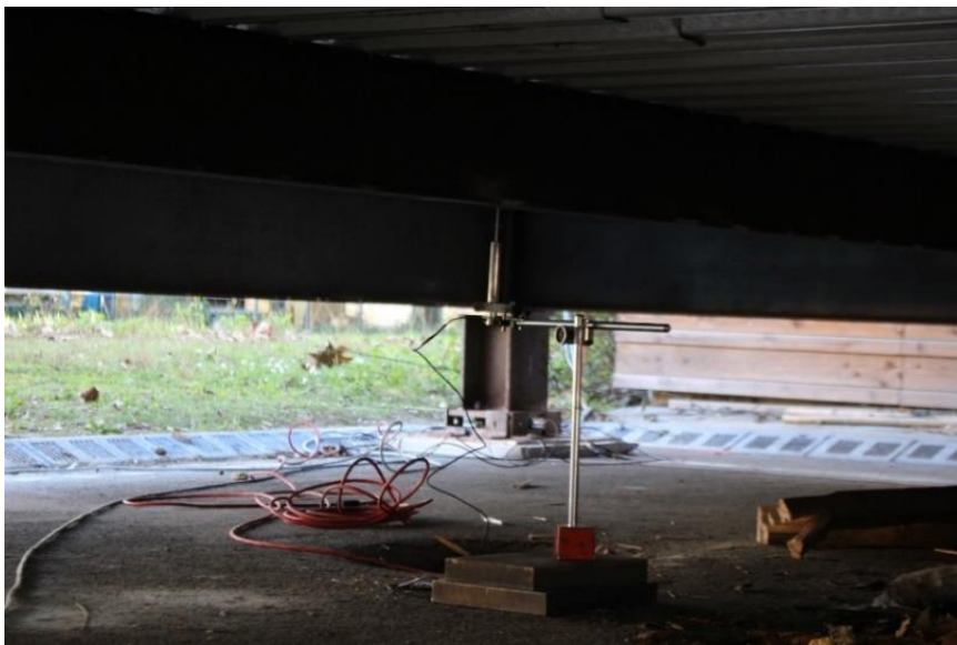
Figure 3.18: LVDT device placed below the floor
