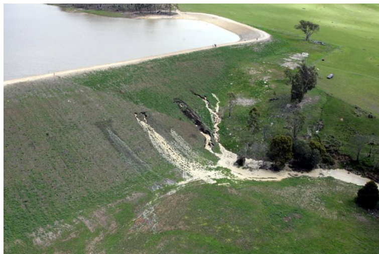
Fig. 1. Failure by piping, Tunbridge dam, Australia in 2005 (available from Geoengineer.org website)
