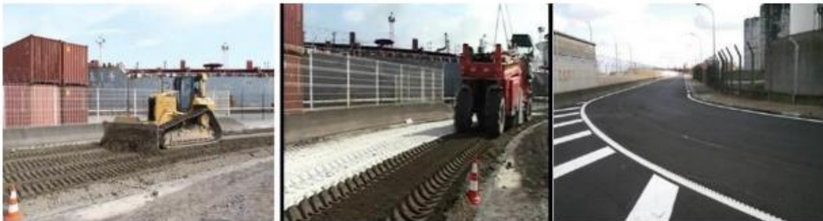
Figure 19. Implementation of the Freycinet 12 road based on dredged sediments at GPMD (Achour 2013).
