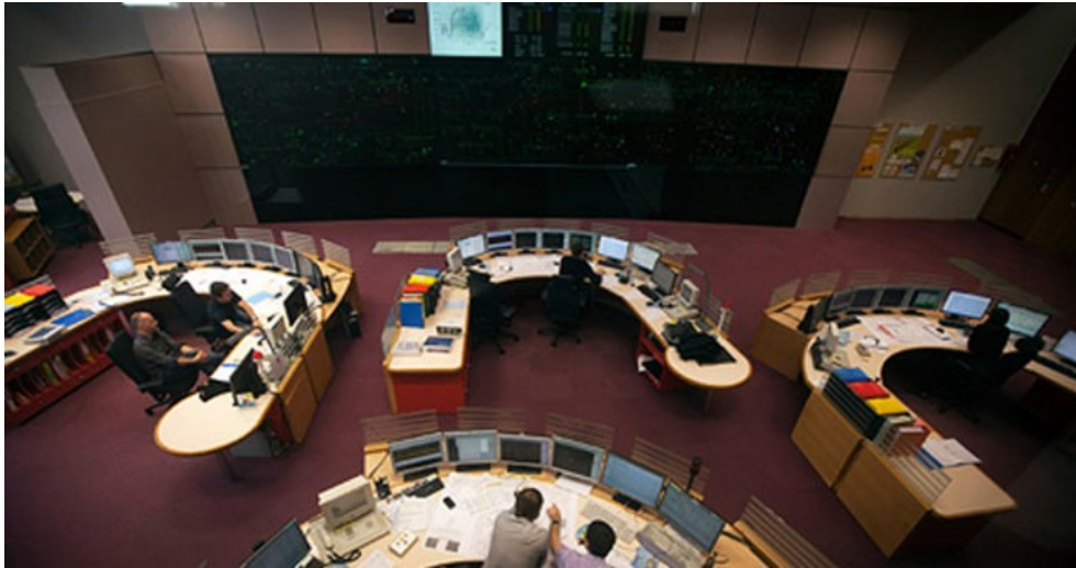
Figure 3.1. RTE's control room
