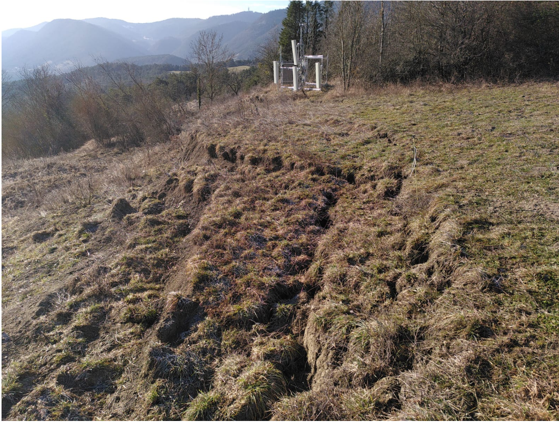
Winter image of the Harmalière RFID measurement station. In the foreground, the first meters of damaged soil that constitute the landslide scarp.
