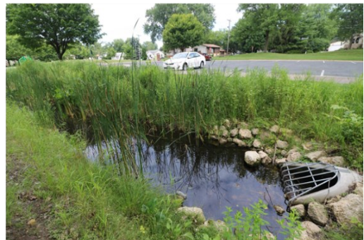
LaBelle Pond bioretention basin, Mississippi, USA
