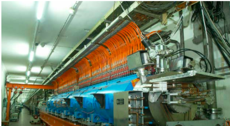
Figure 2.7: Positron focusing and accelerating systems at BEPCII [6].
