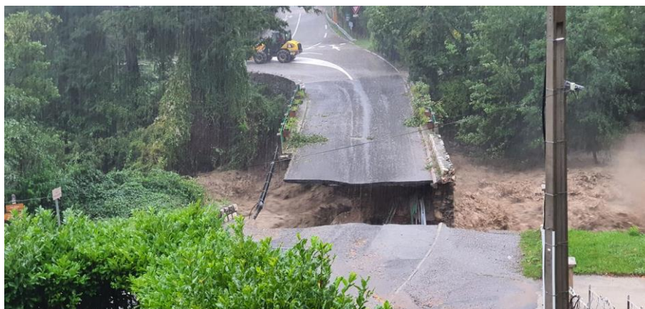
Figure 2-14. The bridge destroyed during Storm Alex. (source: Météo-Paris (2020))
