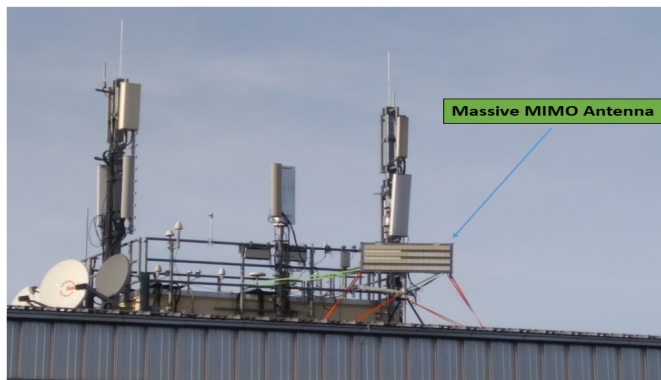
(b) BS antenna with 64 antenna elements is shown here.
