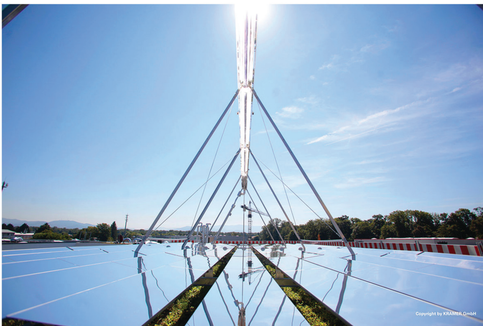
Figure 4. Linear Fresnel collector used to drive an absorption refrigeration system at Umkirch, Germany. (© 2012, suncooling GmbH, a member of the KRAMER GROUP, Germany. Used with permission.)
