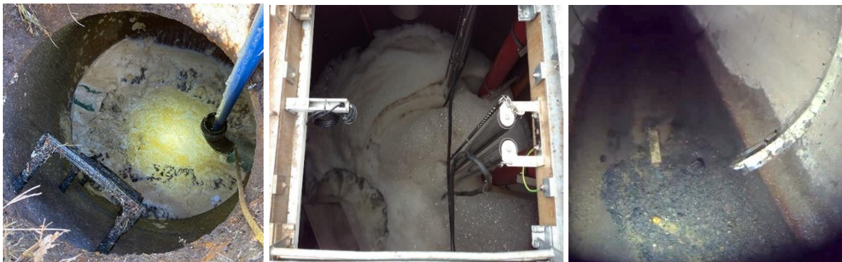
Figure 0-2: Sensors installed in wastewater network.
