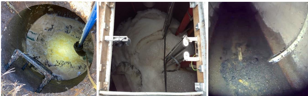
Figure 0-2: Sensors installed in wastewater network.
