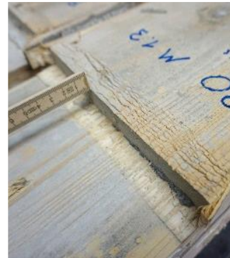
iii. Failure mode
