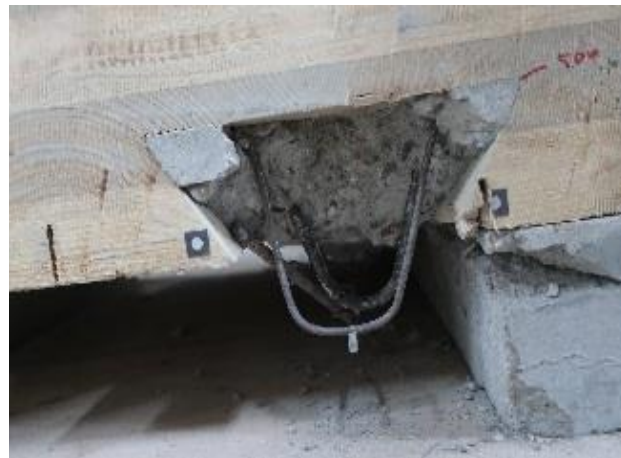
Figure 10: Steel rebars in the concrete notched connectors after collapse (concrete was removed by a jackhammer).
