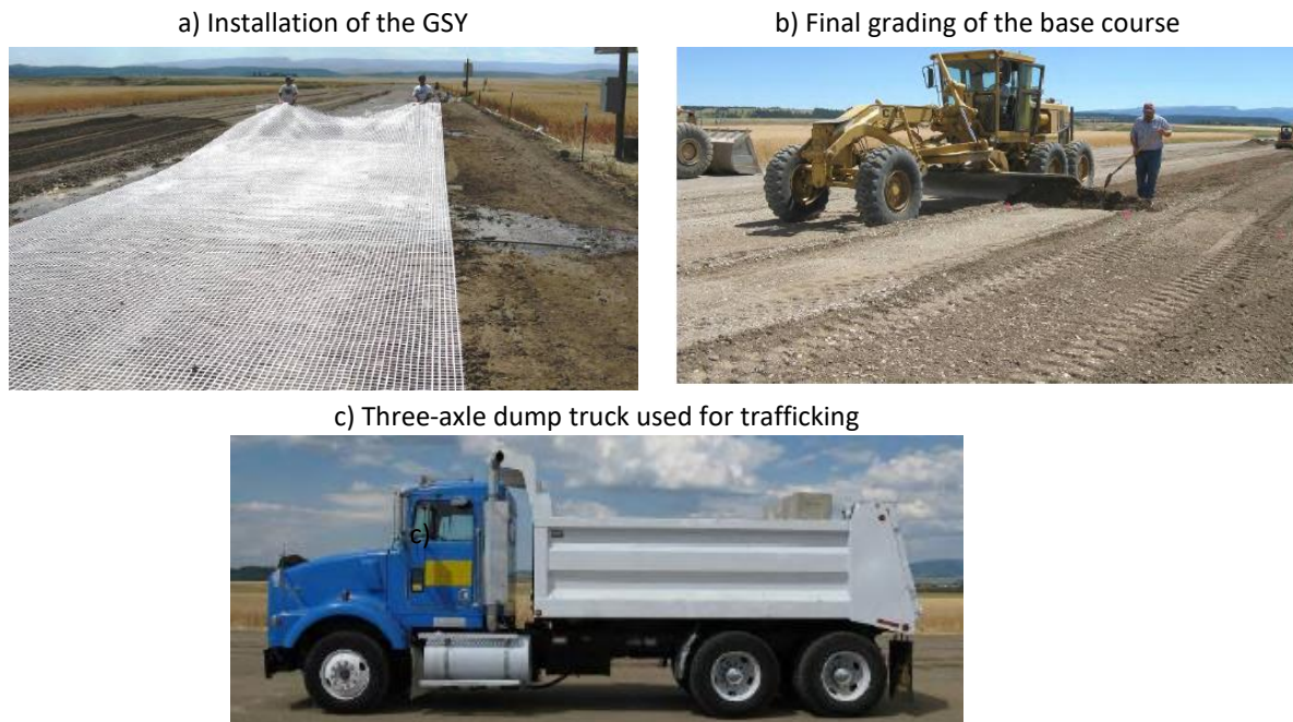
Figure 2-16: Overview of construction procedure of unpaved test pit and the three-axle loading truck (Cuelho and Perkins, 2009)
