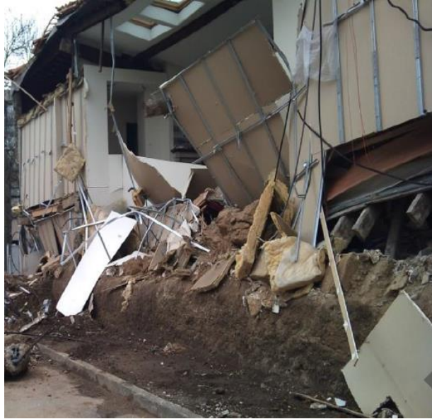
Figure 1.6: RE structural collapse due to water accumulation at the wall base, Lyon, France [33].
