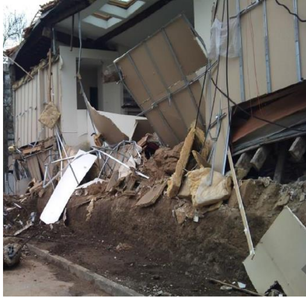
Figure 1.6: RE structural collapse due to water accumulation at the wall base, Lyon, France [33].
