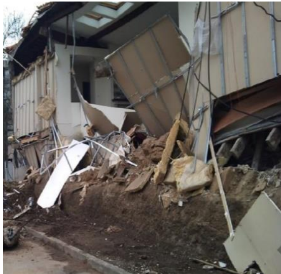
Figure 2.10: Failure of an earth building in Lyon (France), which was produced by a large increase of water content at the wall base, by Scarato and Jeannet (2015) [94].
