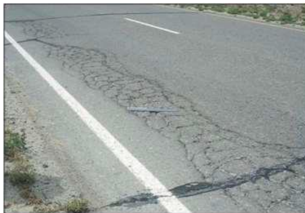
Figure 2.22 – Severe fatigue cracking (Miller and Bellinger 2014) as cited by (Orozco, 2020)
