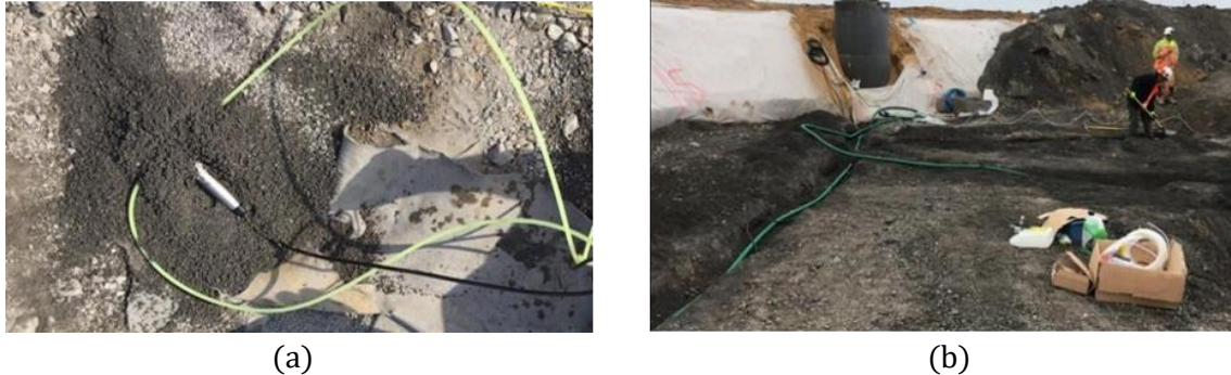
Figure 3-8: (a) Hydraulic transmitters installed at level of the RI, (b) wiring to the acquisition units.
