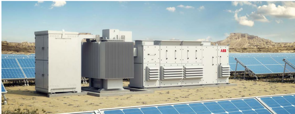
Fig. 2.4. Central inverter on site [11]
