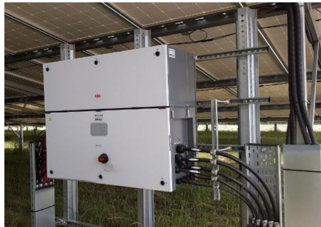
Fig. 2.2. String inverter [9] on site
