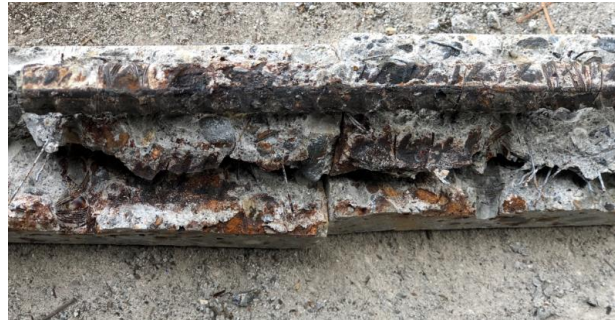
Figure 183. Picture of imprint of corrosion in the SCI of a top bar (with AC)
