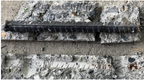
Figure 182. Picture of imprint of corrosion in the SCI of a bottom bar (with AC)
