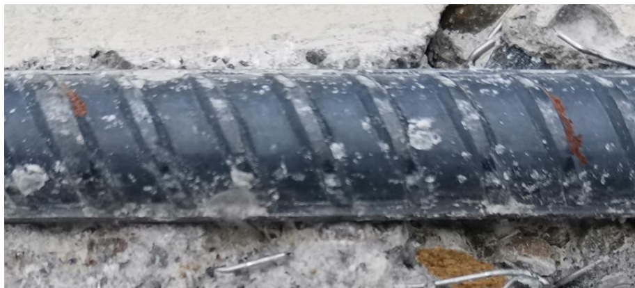
Figure 213 : corrosion visible at the foot of 2 ribs on bottom front bar G3-07 after 30 cycles
