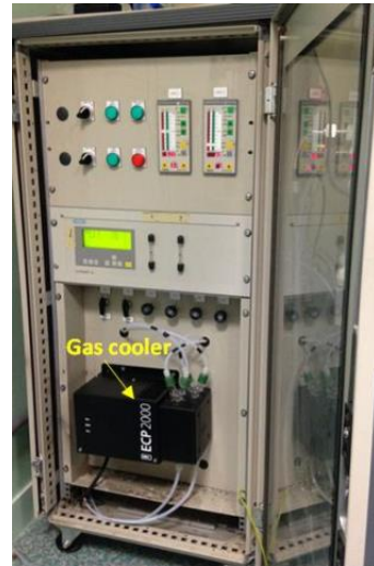
Figure 43. Siemens cabinet of CO 2 analysis and control
