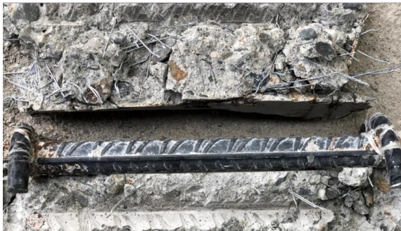
Figure 184. Picture of imprint of corrosion in the SCI of a bottom bar (without AC)
