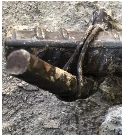
Figure 175 : Example of corrosion on stirrup
