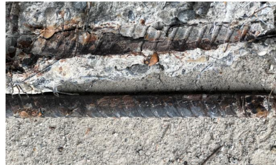
Figure 185. Picture of imprint of corrosion in the SCI of a top bar (without AC)
