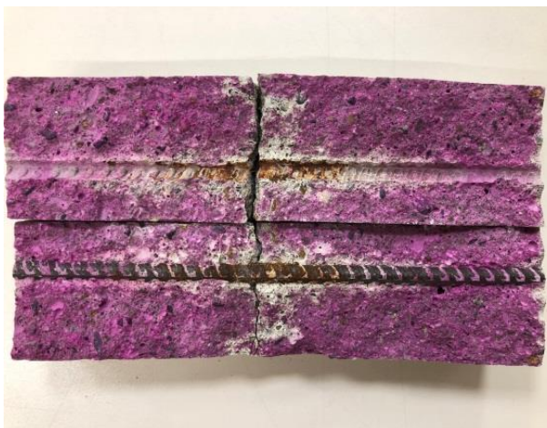
Figure 116 : Carbonation along top bar for ref 3 sample
