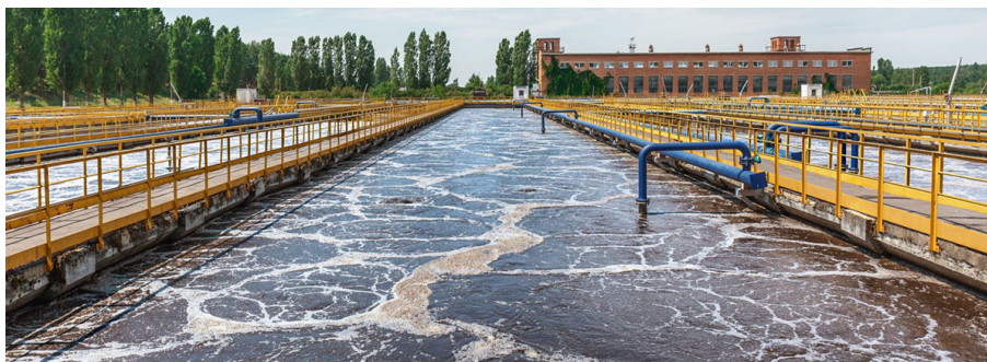
Figure 1 – Aerated pond in an activated sludge wastewater treatment plant. Source: https://cpe.rutgers.edu/water-wastewater/microbiology-of-activated-sludge
