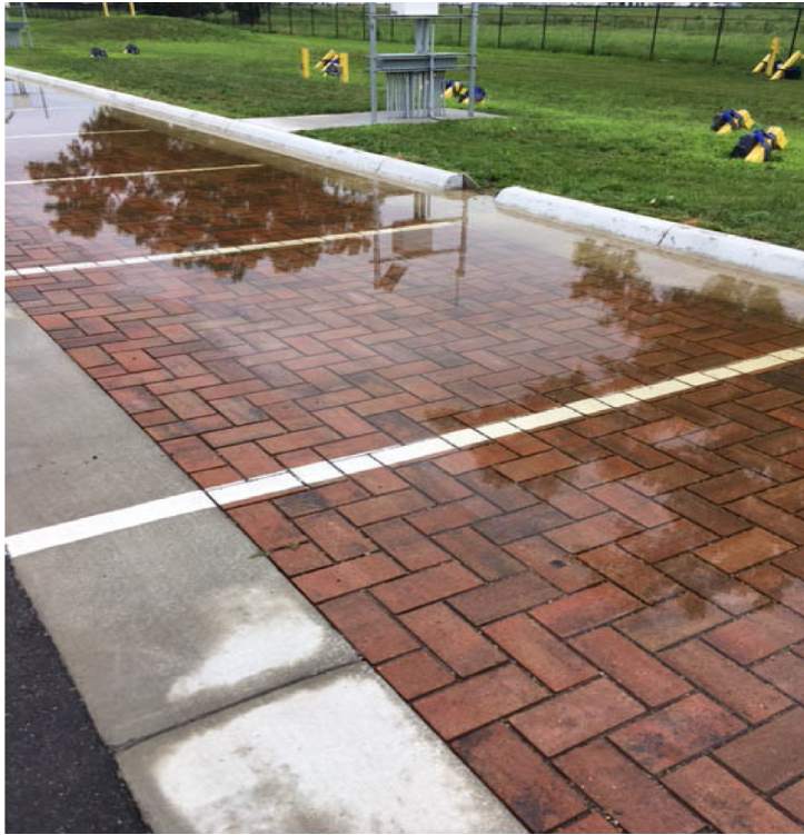
Figure 1.1: Standing water over PICP (permeable interlocking concrete pavers) section after progression of clogging [7].
