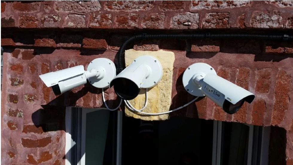
Figure 10. Example of VMS cameras installed in Etretat (picture of Y. Soufflet 2018)
