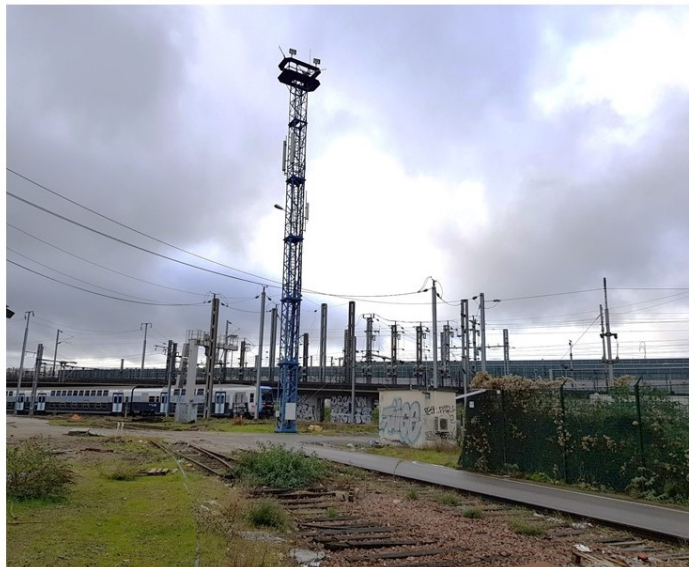
Figure 5.1: A passing train in the railway infrastructure with a GSM-R base station situated next to the railway track. (SNCF Reseau Paris, France)
