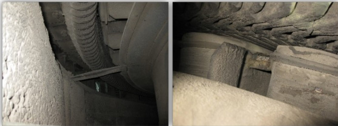
Figure 4.30: Photographs taken during a visual inspection. The photos show a high contamination level.
