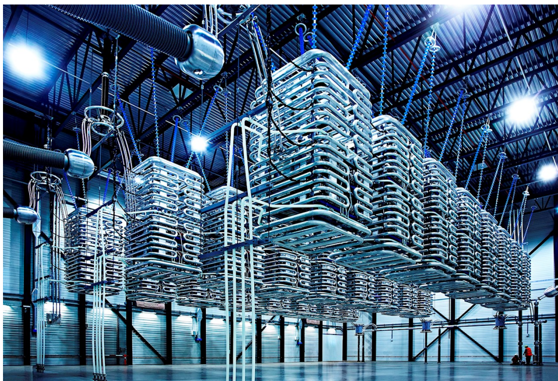
Figure 1.3: An HVDC converter station [3]
