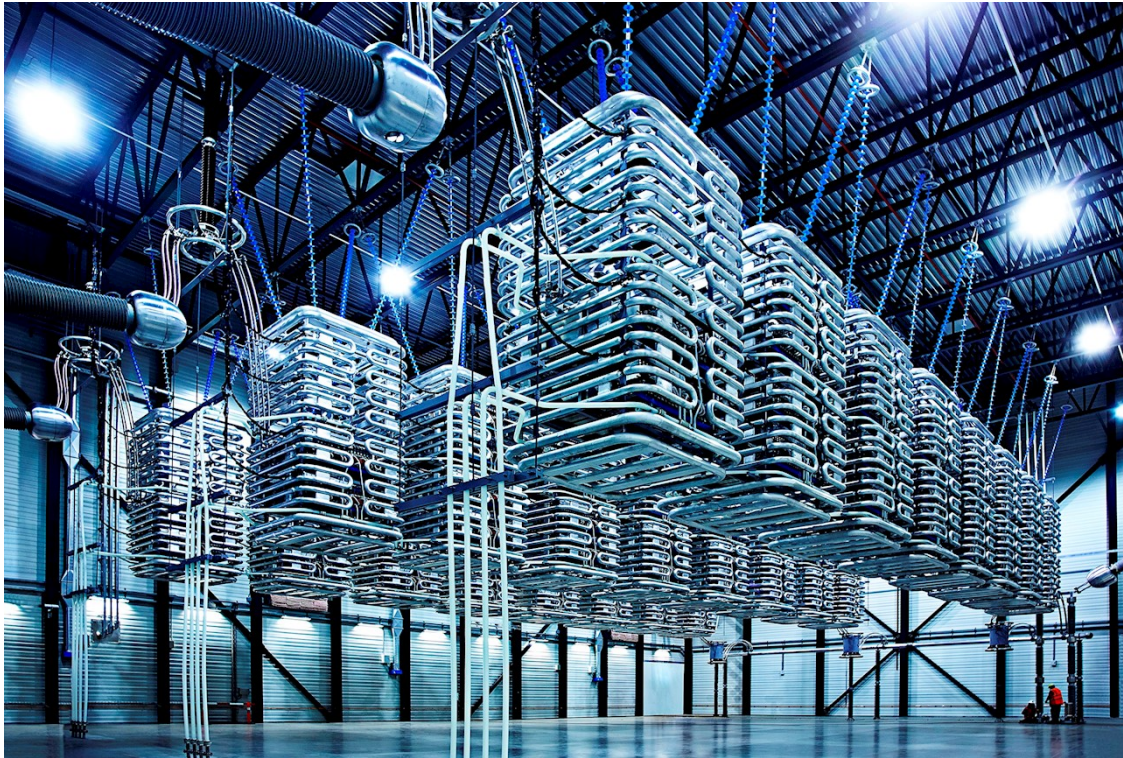
Figure 3: An HVDC converter station [3]
