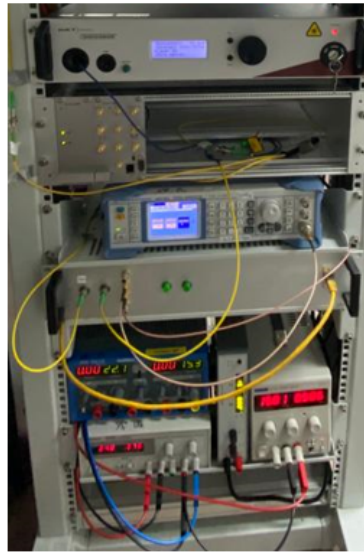
Figure 4.5: Power supply distribution for optical fiber link that includes a combination of four linear power supplies, supplying \pm 15 V, +15 V and +12 V with a total weight of 25 kg and occupying a dimension of approximately 5U.
