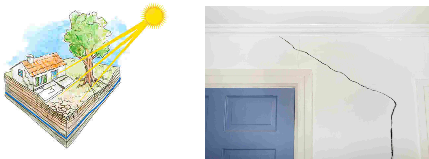
Figure 2.3 – Left: the clay shrinking-swelling phenomenon. Right: an example of crack due to the clay shrinking and swelling phenomenon.
