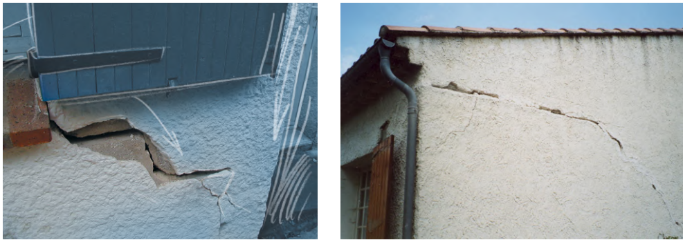
Figure 1.8: Two examples of building damage caused by clay shrinkage or swelling (photos of BRGM)
