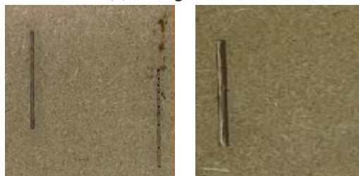
(c) Rectangular cracks
