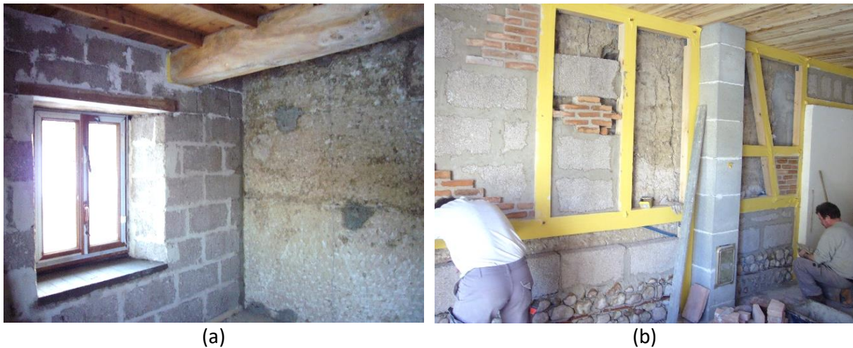
Fig. 2.6: Interior finishing plaster layer of traditional rammed earth buildings chopped off before retrofit.
