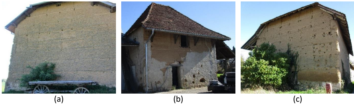
Fig. 4.9: Erosion damage by wind-driven rain: (a) edge erosion breaks, frost damage ( Appendix B ); (b) frost damage and erosion; (c) invigorated damage around impermeable hard gravel.
