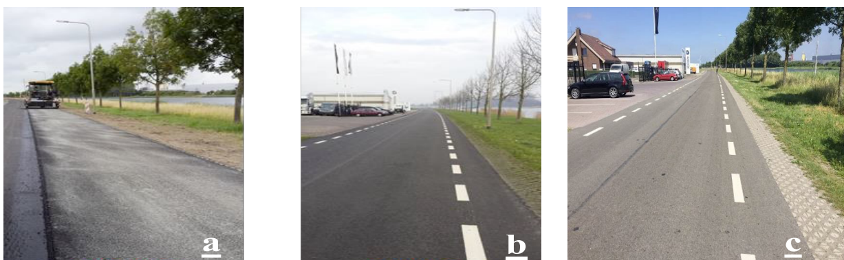
Figure 14: Example of road demonstration of bioasphalt mixed with conventional one in Zeeland, southwestern Netherlands. The pictures showed (a) the start of putting the mixture on road in 2015, (b) how the road looked in 2015 and (c) in 2019.
