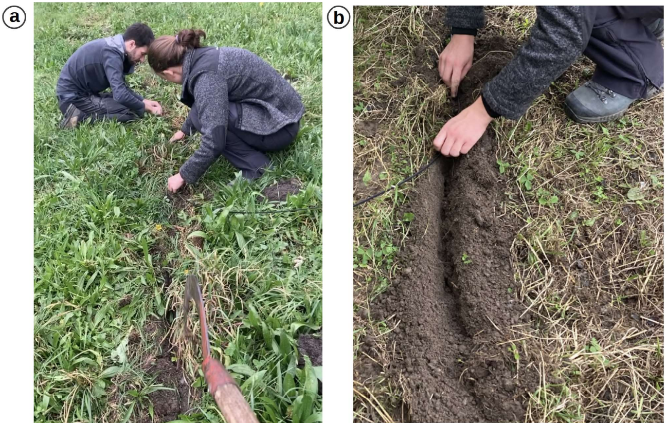
FIGURE C1.2: Viella field work. (a) shows making a furrow with a hoe, (b) shows putting the fiber optic cable inside the furrow.
