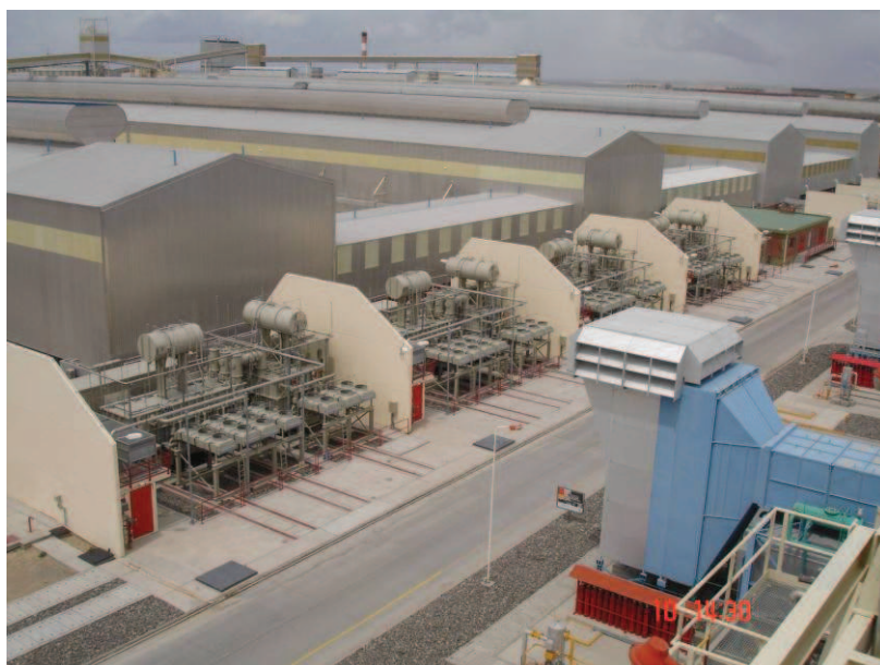
Figure 10. Example of an Alstom Grid AC/DC conversion substation (Aluar, Argentina)
