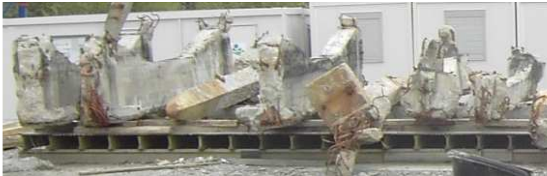
Figure 6.6 — Beams after 80 years of exposure.
