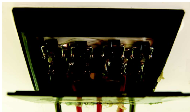
Figure B.5: The junction box with the bypass diodes
