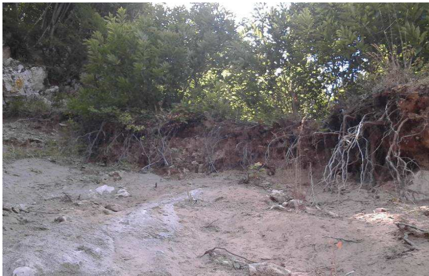
Figure 30 – Roots that failed by pull out in a previous landslide in the region of Campania.
