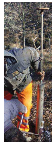
Figure 99 – Tube and extension used to open a borehole for the installation of TDR probes.
